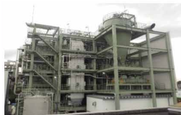
Tamagawa Joryu Water Reclamation Center Stoker Incinerator
