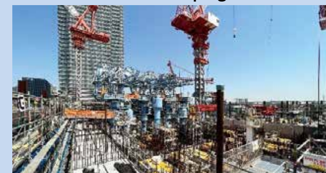
Koto Pump Station
