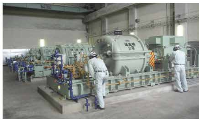
Blower inspection (Kita-Tama Ichigo Water Reclamation Center)
