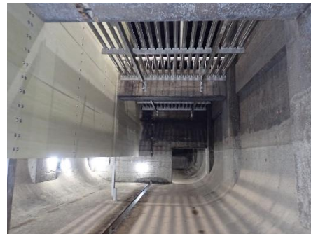
Semi-advanced Treatment Facility (Kiyose Water Reclamation Center)
