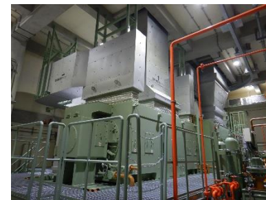
Power Generation Facilities After Reconstruction (Umeda Pumping Station)
