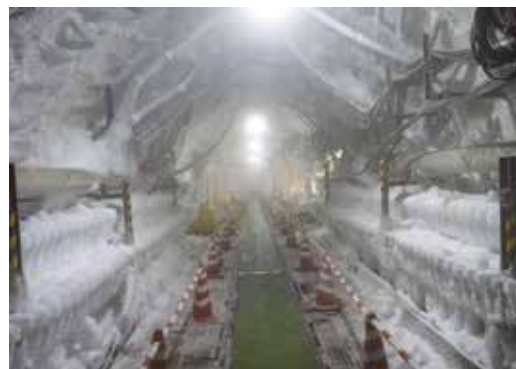
Fig.11 Inside the pipe in freezing
