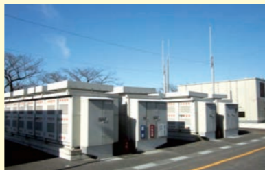
▲ NaS (sodium-sulfur) Battery
