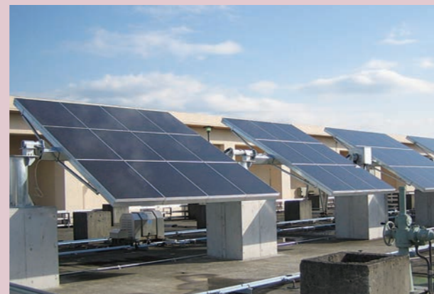
▲ Single-axis tracking type photovoltaic cell
