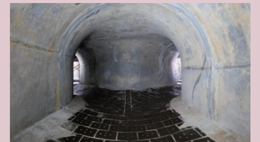
▲Pump well connection
