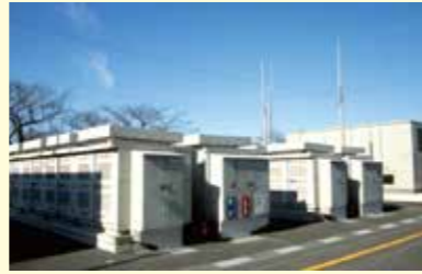
▲ NaS (sodium-sulfur) Battery
